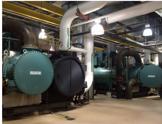
The Central Chiller Plant
