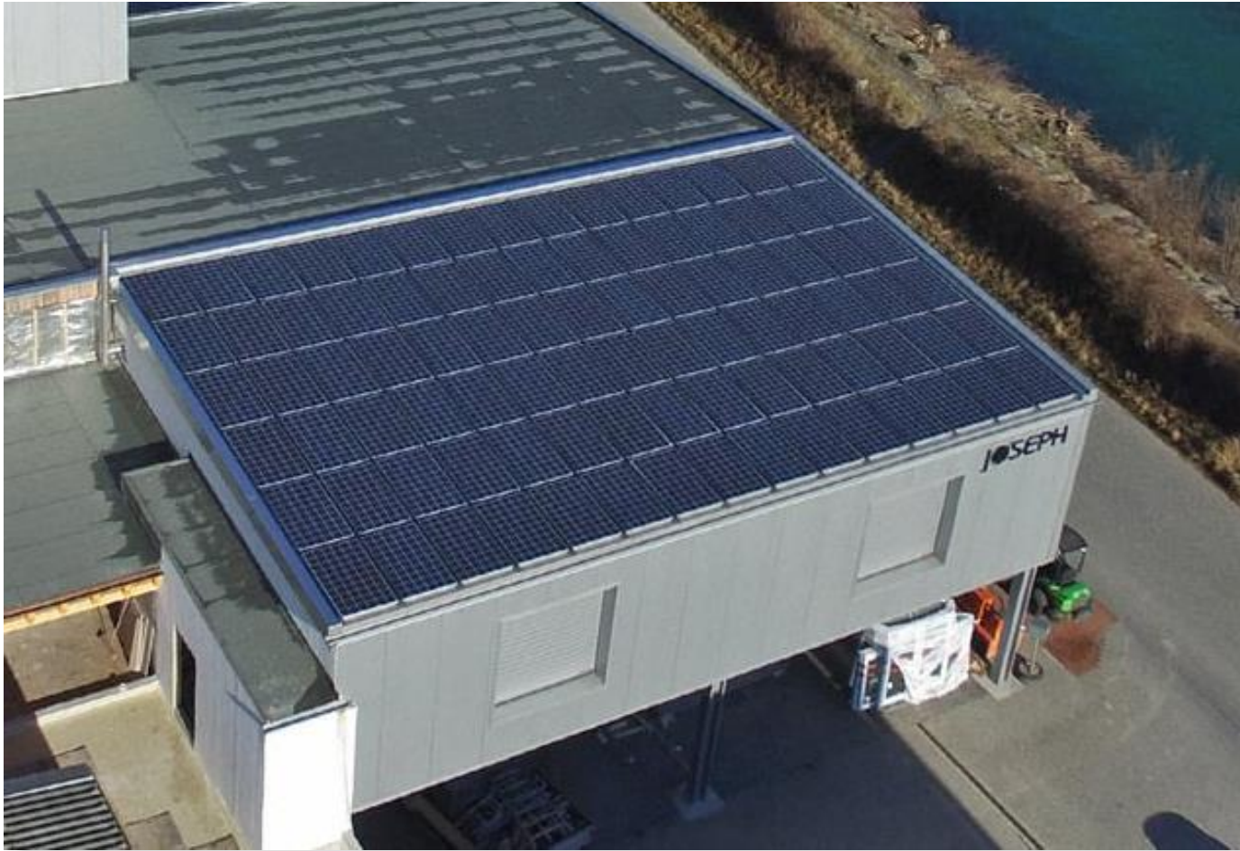
170 sqm, 23 kWp, Switzerland - Warehouse
